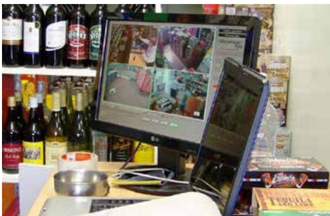
Example of CCTV monitor
