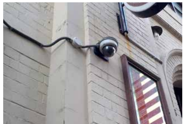
Example of CCTV surveillance at the entrance/exit of a bar
